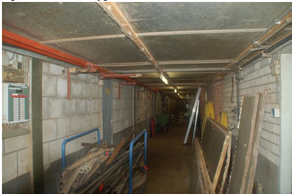
centrale gang stal 3
