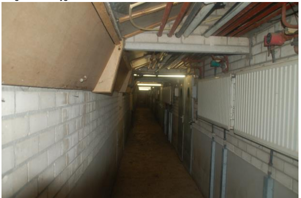
centrale gang stal 1
