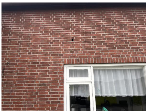
Woning Markweg 5: opening in gevel.
