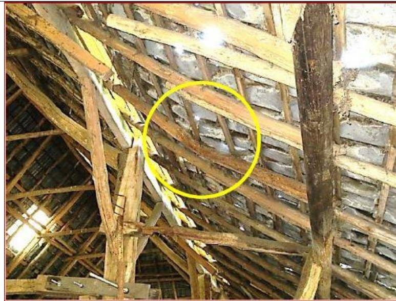
Dak no. 7: spoor gebroken
