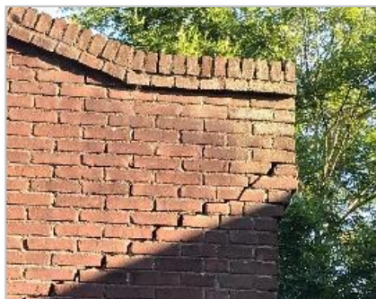
Foto 12: Scheur in pand.
