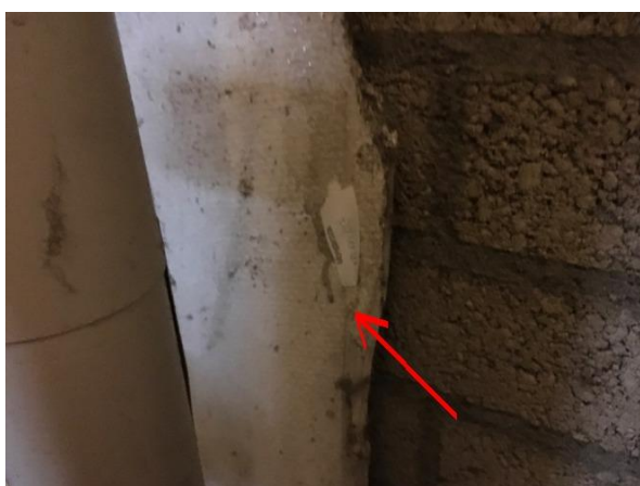
Brandwerende beplating los detail
