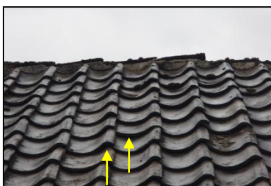
Figuur 12. Opening in dak.
