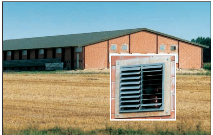
Use of wall fans
