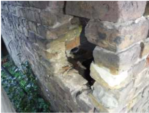
Gaten in gevels woning.
