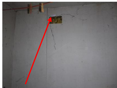
foto: brandwerende beplating (MM6)
