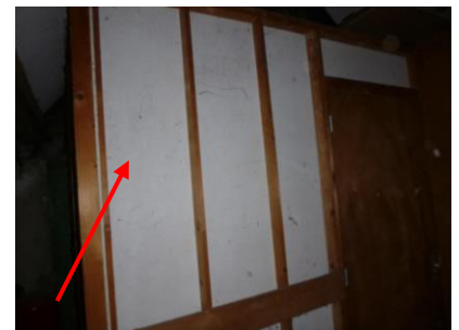
foto: brandwerende beplating
