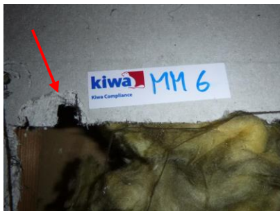
foto: brandwerende beplating (MM6)
