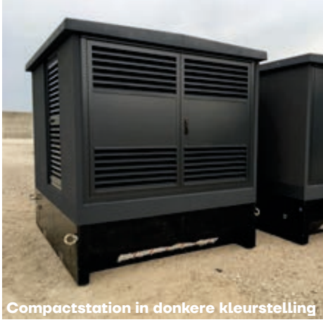
Compactstation in donkere kleurstelling
