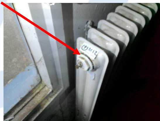
Foto 25 | Pakking lamellen radiator
