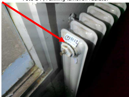
Foto 26 | Pakking lamellen radiator
