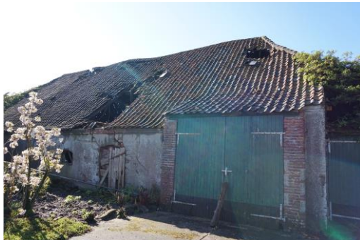
Golwing van nok, lacunes in dakvlak
