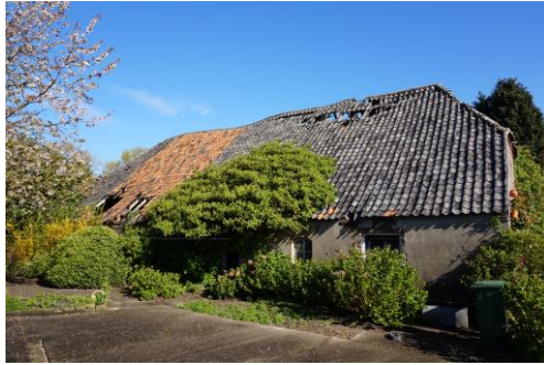
Golwing van nok, lacunes in dakvlak
