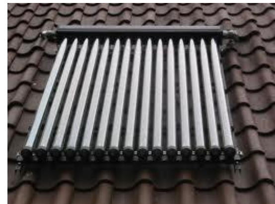
Heatpipes tbv zonneboiler
