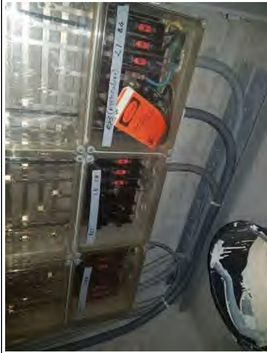
Foto 65: Meszekering in kelder, schacht as 11 (bron 41)
