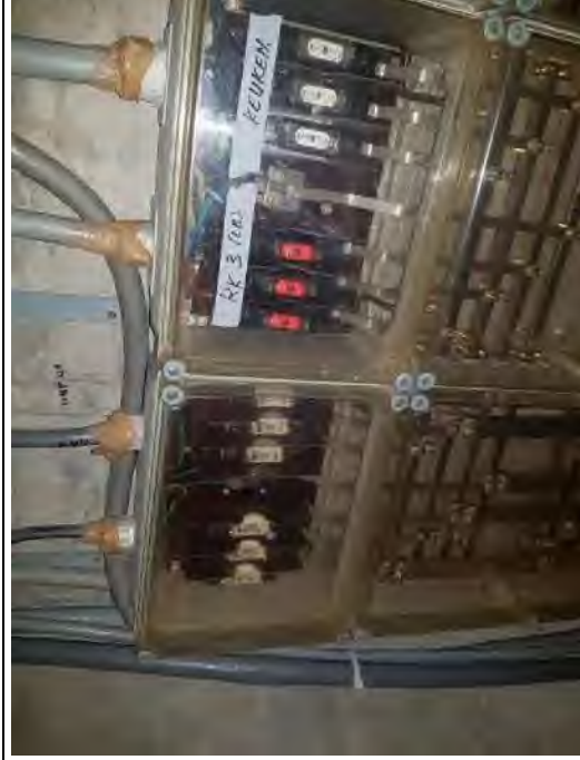
Foto 66: Meszekering in kelder, schacht as 11 (bron 41)
