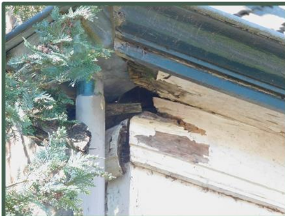
Gat in houten betimmering
