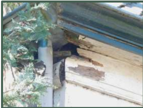
Gat in houten betimmering
