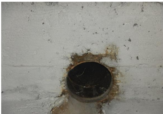
Pvc-buis in schoorsteen
