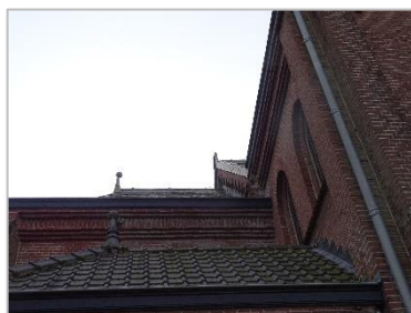
Foto 14: Openingen langs houten dakrand.
