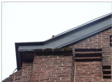
Foto 5: Openingen langs houten dakrand.
