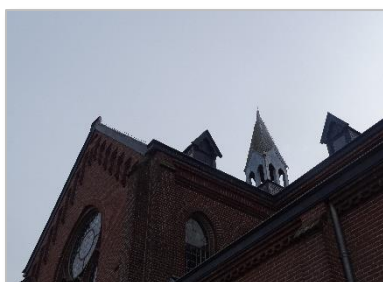
Foto 12: Openingen langs houten dakrand
