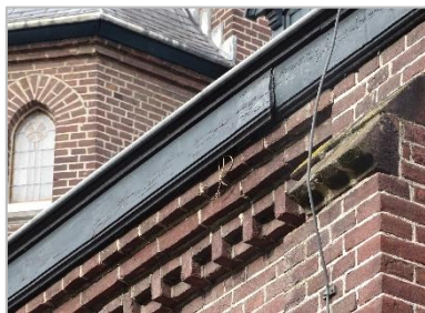
Foto 3: Openingen langs houten dakrand.
