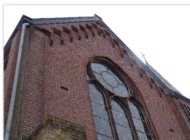
Foto 13: Openingen langs houten dakrand.
