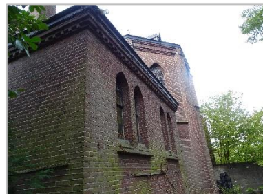
Foto 7: Openingen langs houten dakrand.
