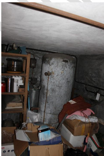
Hydrofoor in kelder
