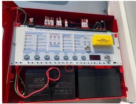
Figure 7-3 Internal of Fire Control Box
