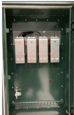
Figure 6-6 APS Power Connection
