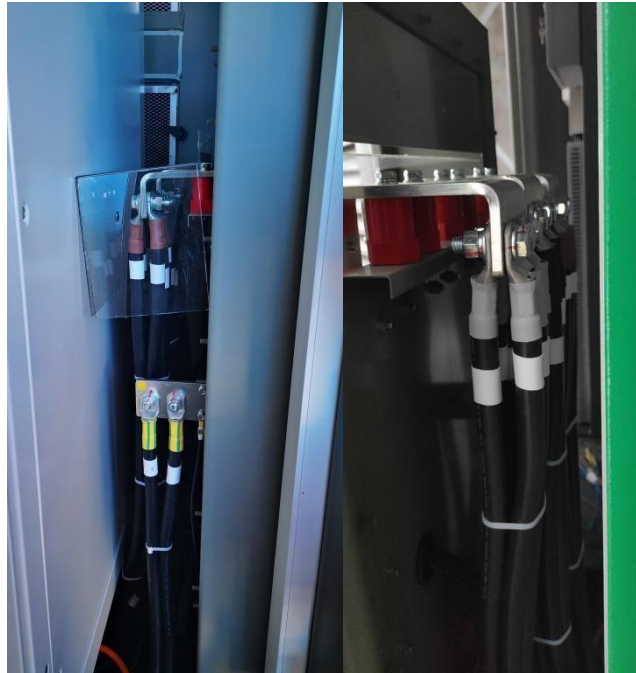
Figure 6-6 Container AC Main Joint
