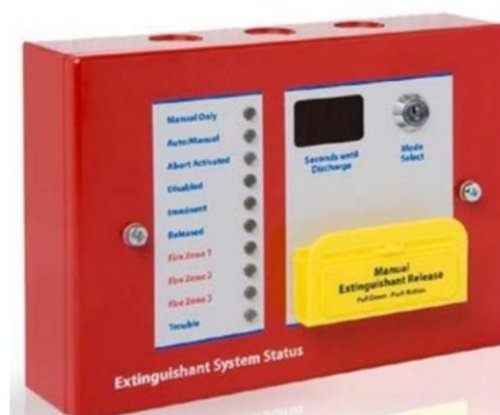
Figure 8-5 Manual/Automatic Switch Box
