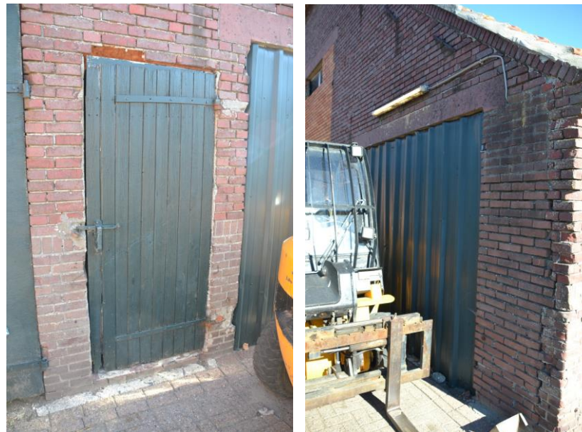
Links: later aangebrachte loopdeur. Rechts: vm. staldeuropening.
