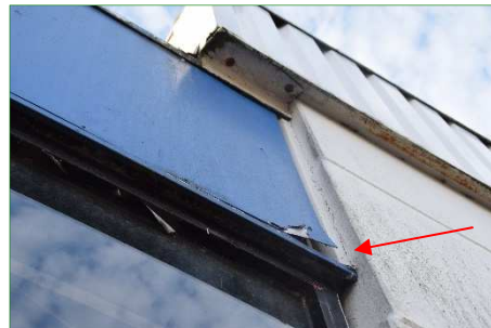
Locatie 3: kier in beplating.
