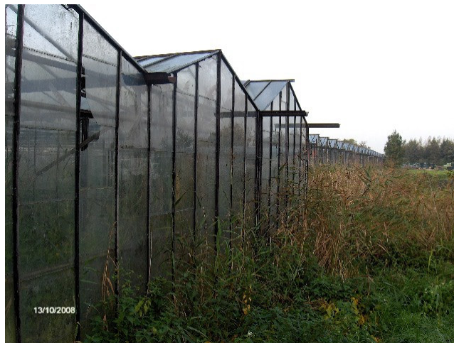
Te slopen kas (asbesthoudende beglazingskit).
