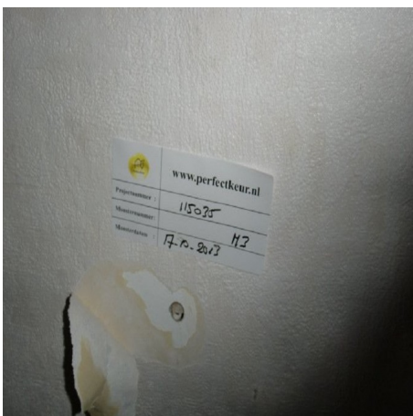
M3 is asbesthoudend.
