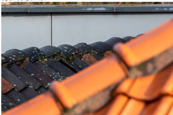
Opening in dakpannen
