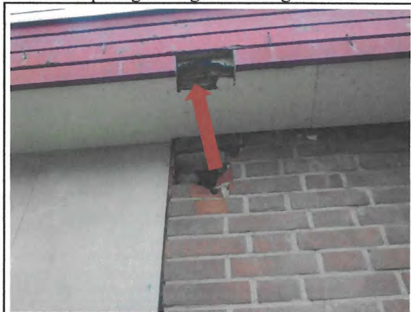
Foto 26: opening in dakgootbekisting
