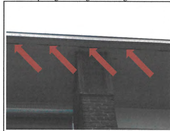
Foto 22: openingen in dakgootbekisting
