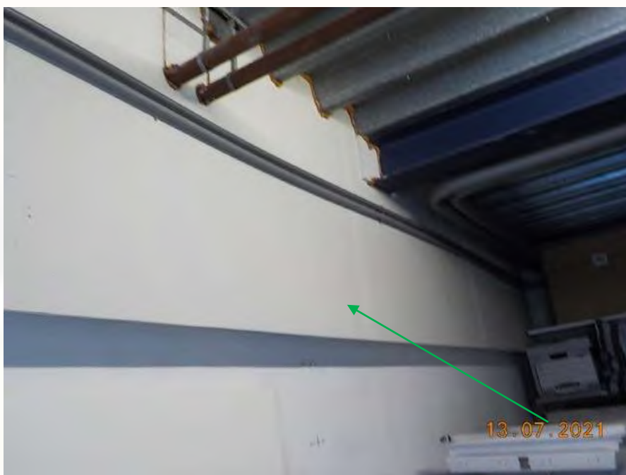
Foto 6: Bron B02, Asbestvrije beplating, brandwering
