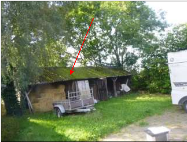
Foto 73: Schuur 4: Golfplaten dak incl. overlap & toebehoren (Bron 7) (Asbesthoudend)
