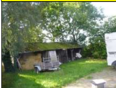
Schuur 4: Golfplaten dak incl. overlap & toebehoren (Bron 7) (Asbesthoudend)
