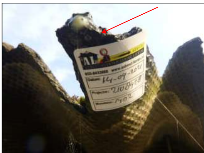
Foto 11: Schuur 1 & 2: Golfplaten dak incl. overlap & toebehoren (Bron 2) (Asbesthoudend)
