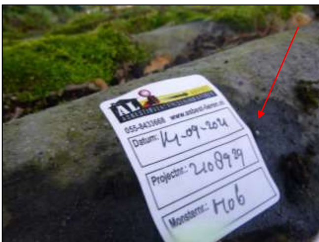
Foto 65: Schuur 3: Golfplaten dak incl. overlap & toebehoren (Bron 6) (Asbesthoudend)
