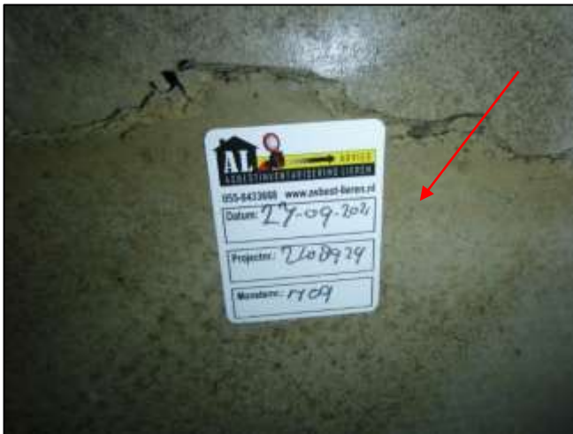
Foto 79: Woning: Dakbeschoot (Bron 9) (Asbesthoudend)
