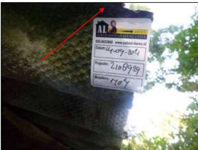
Foto 71: Schuur 4: Golfplaten dak incl. overlap & toebehoren (Bron 7) (Asbesthoudend)
