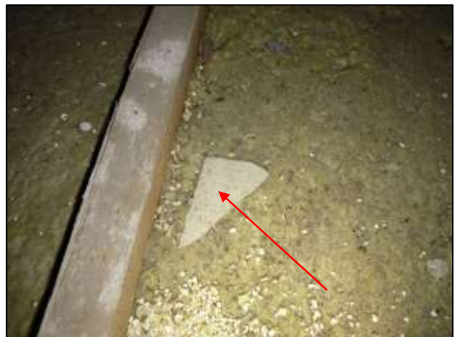
Foto 82: Woning, zolder; Restanten dakbeschoot (Bron 23) (Asbesthoudend)
