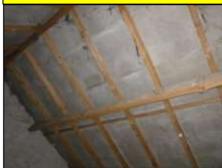
Woning: Dakbeschot (Bron 9) (Asbesthoudend)
