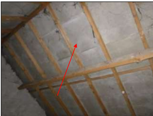
Foto 81: Woning: Dakbeschoot (Bron 9) (Asbesthoudend)
