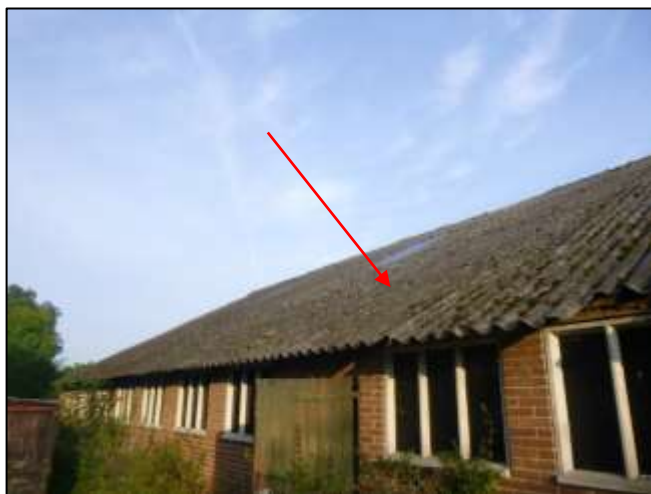
Foto 13: Schuur 1 & 2: Golfplaten dak incl. overlap & toebehoren (Bron 2) (Asbesthoudend)
