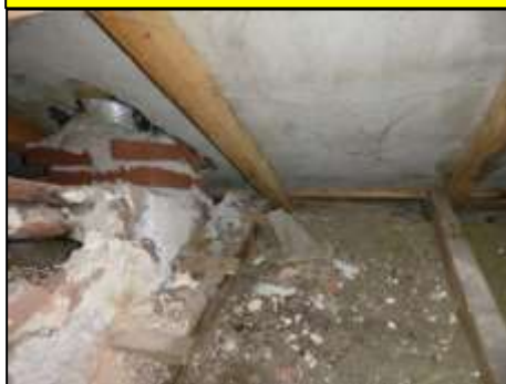
Woning, zolder: Restanten dakbeschot (Bron 23) (Asbesthoudend)
