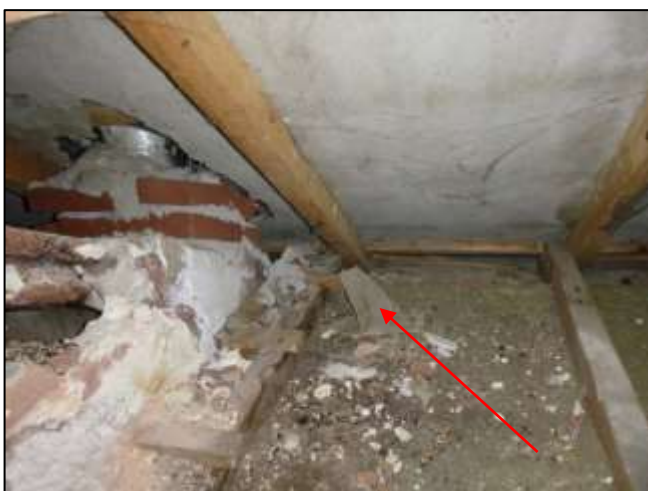
Foto 83: Woning, zolder; Restanten dakbeschoot (Bron 23) (Asbesthoudend)
