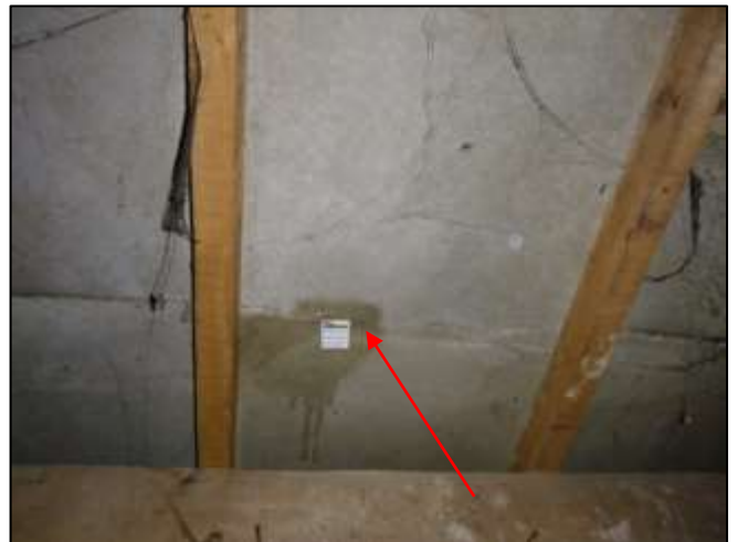
Foto 80: Woning: Dakbeschoot (Bron 9) (Asbesthoudend)
