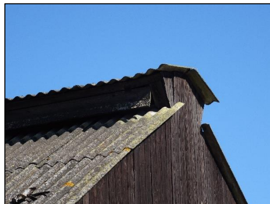
Fig. 2.10 Wijkende planken in nok (bron: FF Solutions)
