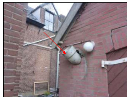
Foto 17: Garage: Buis (Bron 12) (Asbesthoudend)
