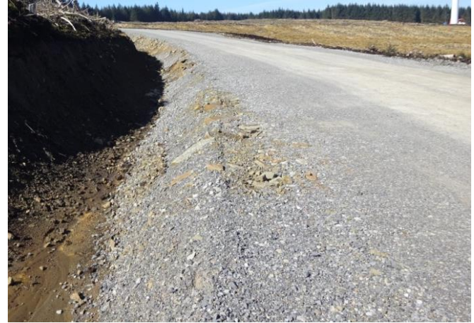
Figure 3: Example of a well groomed gravel road with a slope for proper drainage.
