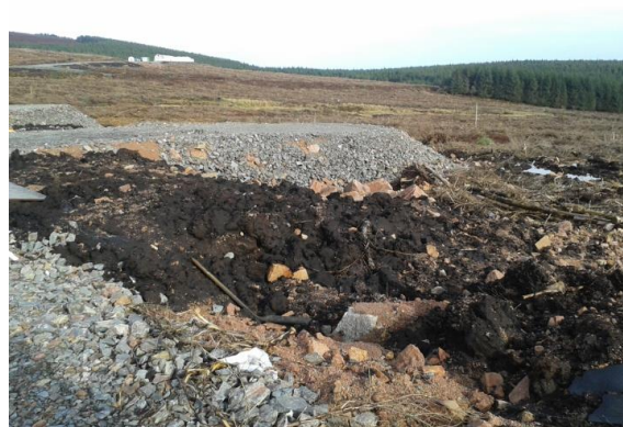
Figure 20: Example of an unacceptable/unprepared area between blade fingers.
