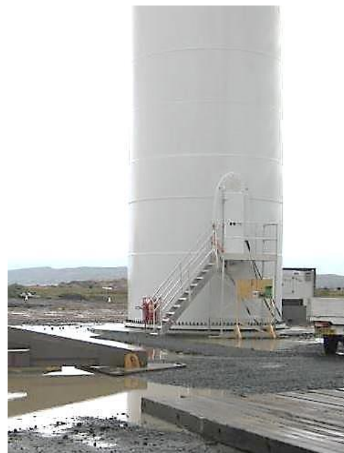
Figure 26: Example of not well-maintained service access to WTG.
