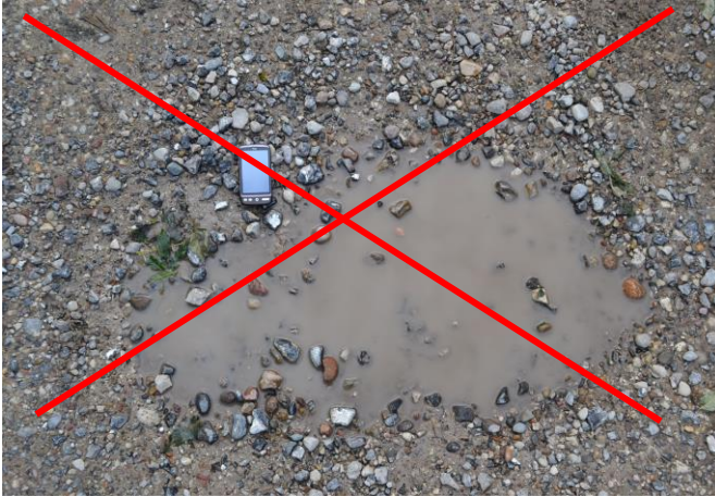
Figure 2: A well maintained Site Road shall not have potholes deeper than 30mm and/or a distribution/collection of potholes that at the reasonable discretion of the Contractor cause unsuitable or unsafe driving conditions.
