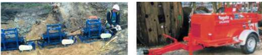
Figure 17 Typical cable tensioners (left) & cable winch (right)
